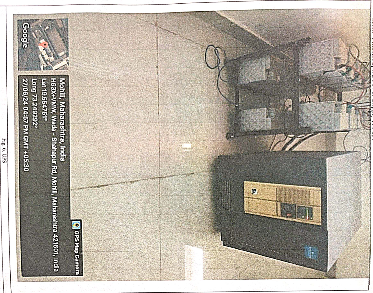
4.3.1.1 Uninterrupted Power Supply (UPS) 1
